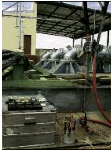
View over the head of No. 2 shaft of the abandoned Berg Aukas Mine: Four strong submersible pumps of which each has a capacity of 360 m 3 /h were installed in the shaft in 1997 to lift groundwater from the open underground mine workings and the dolomitic host rock. The four pumps can be run simultaneously, but presently the set-up is two production pumps and one stand-by pump.
